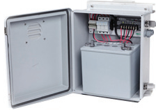
30 Watt solar power supply with 55AH battery; Div 2
